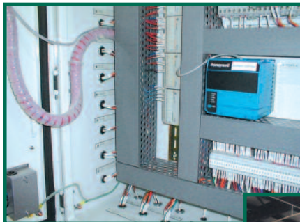
Advanced Electrical Control Panels
