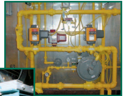
Gas Valve Train
