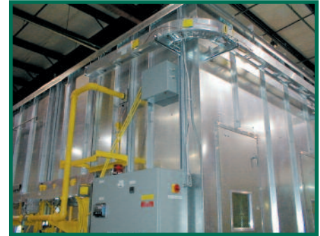
Cabling Systems (Optional)
